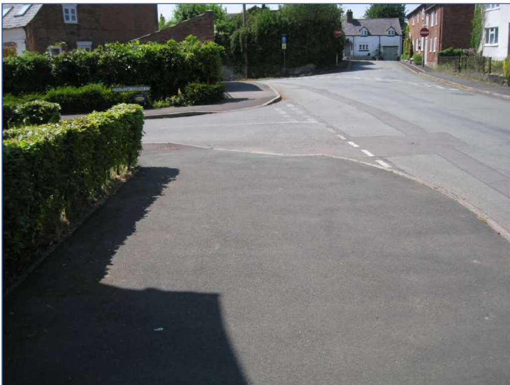
Photo 12 – Church Close dropped kerbs
