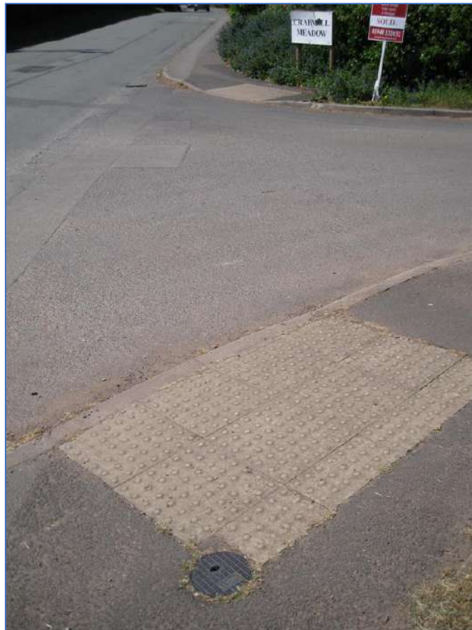
Photo 7 – Misaligned tactile paving at the Tilstock Road / Crabwell Meadow junction
