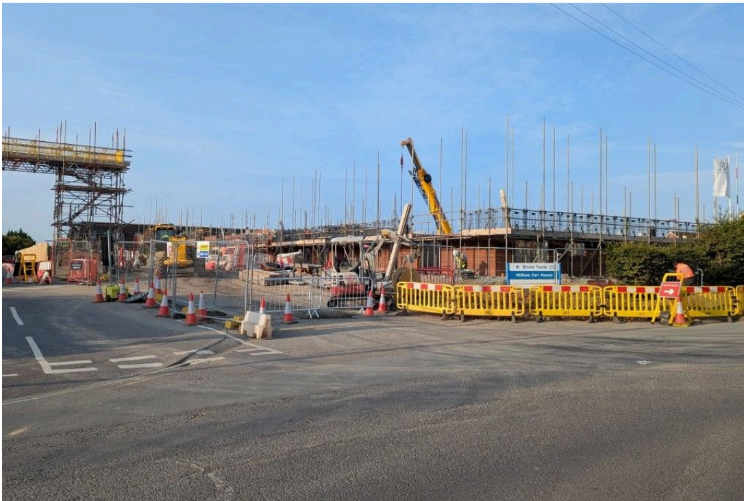
The brownfield site at William Farr House is being redeveloped to provide extra-care affordable housing. Photo: Shropshire Council
