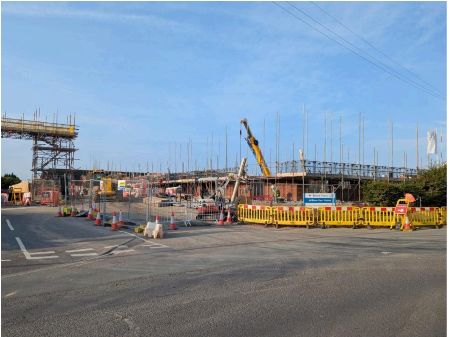
The William Farr House, a redevelopment of brownfield site to provide extra-care affordable housing
