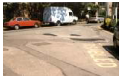
Plate 52: Patchwork of tarmac cadam, St Mary's Place
