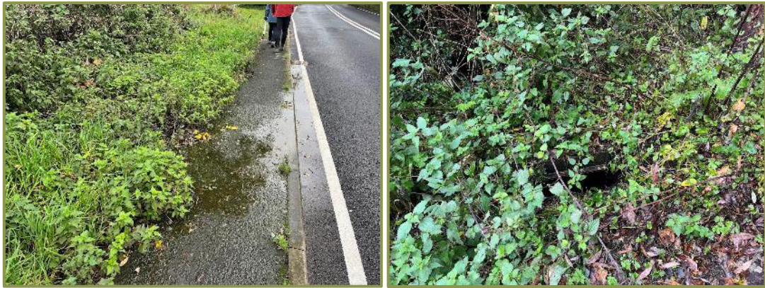
Left: Surface Water Flooding onto the pavement of the A464, and the A464 itself. Right: Open manhole that is connected to Ditch 3
