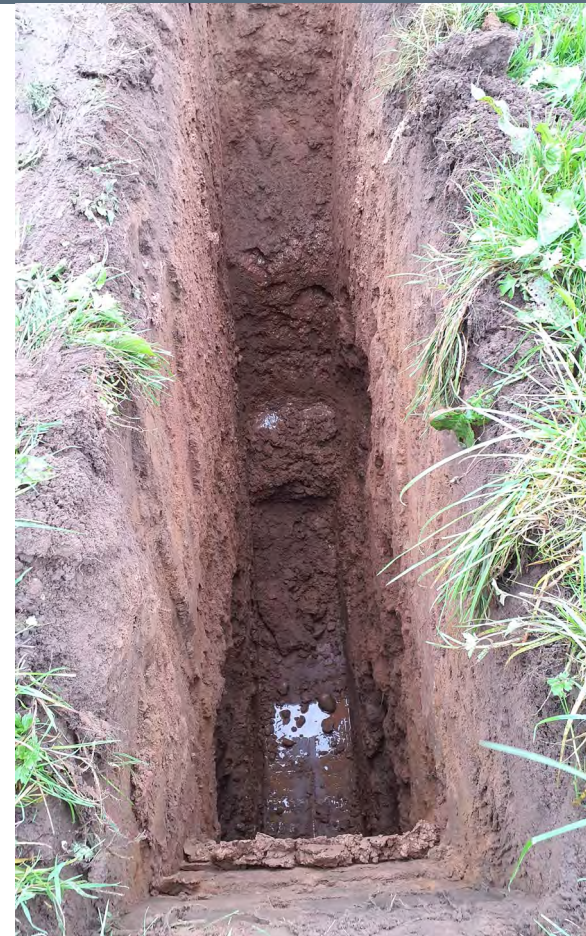
TP07: Showing water ingress and running sand
