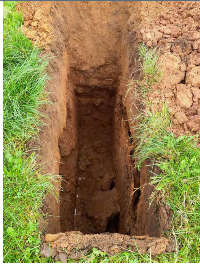
TP04: Showing side wall collapse and water ingress.
