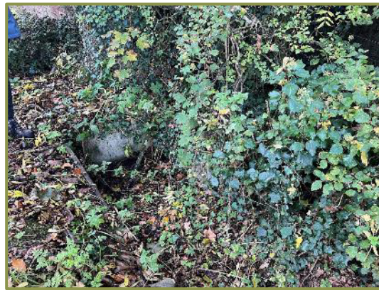
Bottom: Blocked trash screen at the southern end of the ditch.
