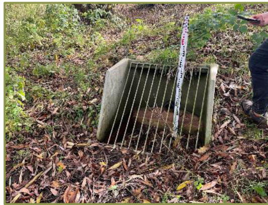
Trash Screen with black pipe that is situated southeast of Pond 2.
