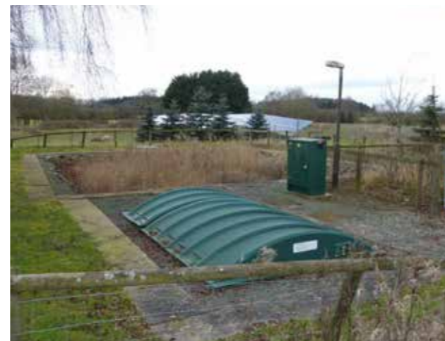
Sustainable drainage facilities such as reed bed systems will form part of the design.
